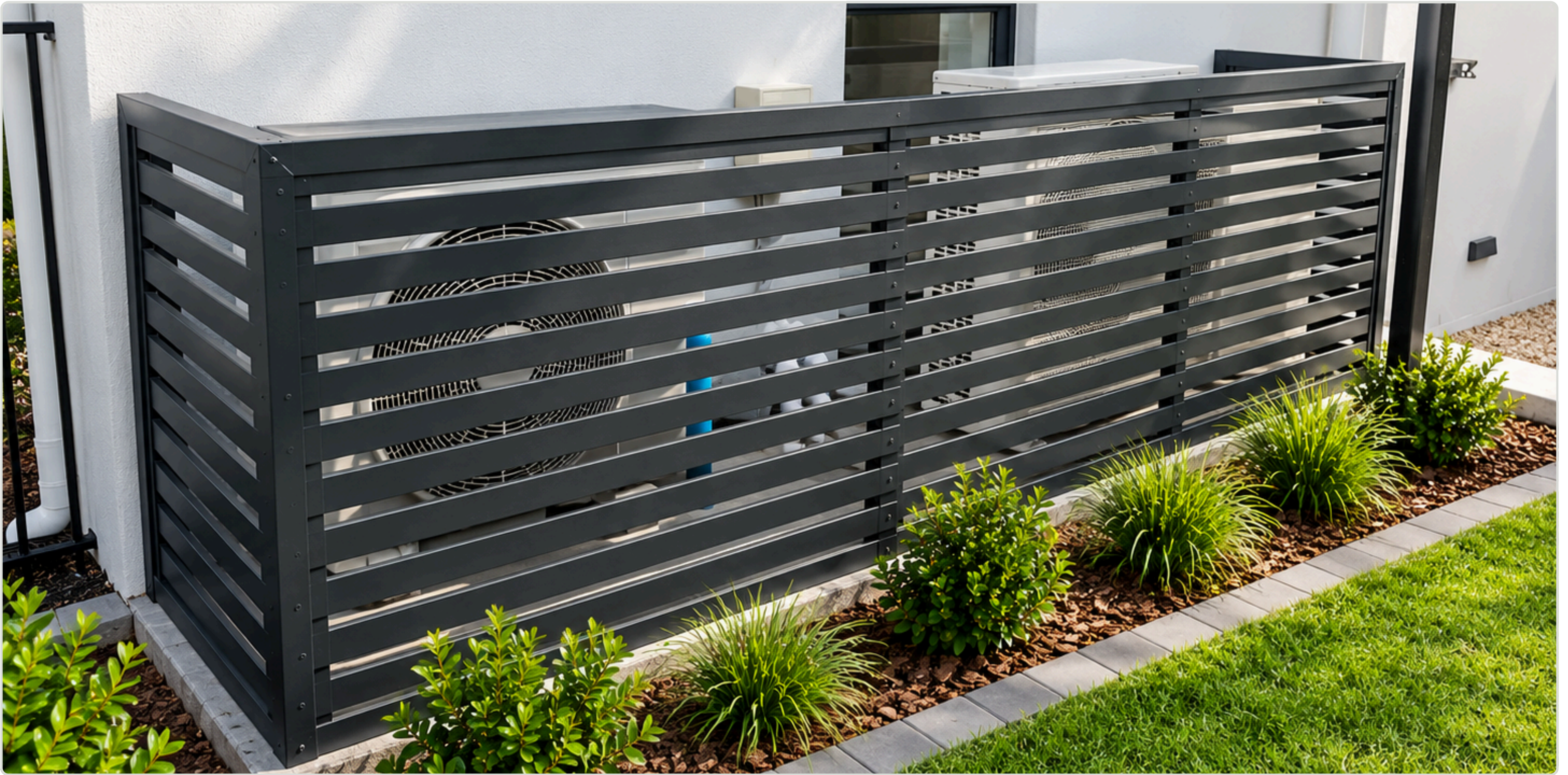
Custom aluminium screening | Purpose-built aluminium screening conceals external air-conditioning units, keeping services accessible while maintaining a clean, considered exterior.
